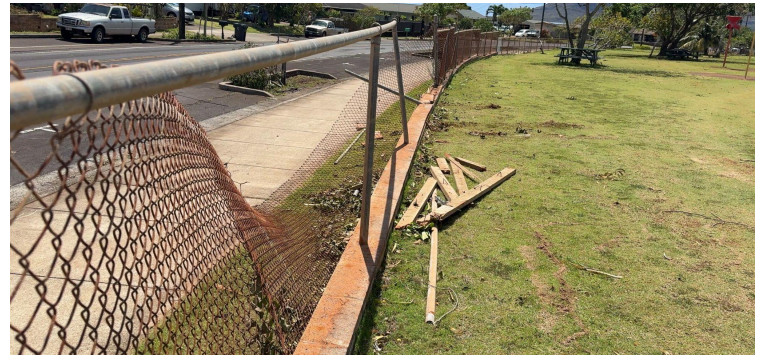
Damaged fence line at Elsie H. Wilcox Elementary in Līhu'e.
