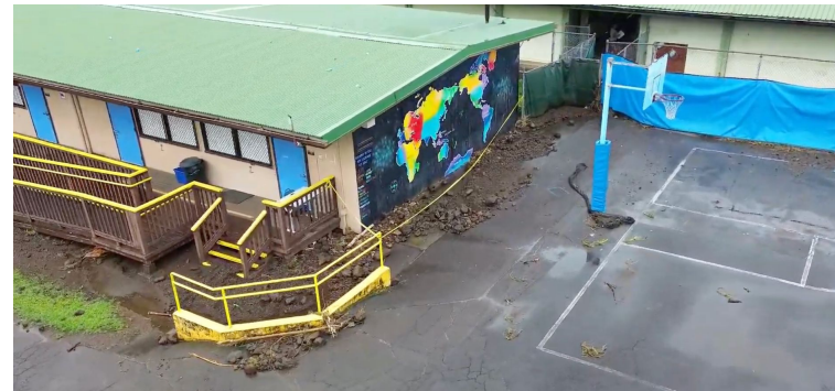
Flood damage at Konawaena High.
